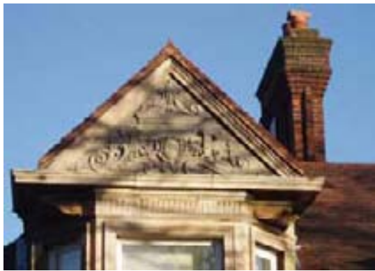
No. 105 has highly ornamental stone dressings: the two-storied bay has elaborately moulded architraves and is surmounted by a gable filled with decorative scrollwork and a cartouche, below which is a frieze with reeded mouldings and scrolled consoles. The property also has wide corbelled brick chimneys
