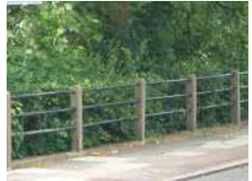
Figure 87: & Figure 88: Post-&-Rail fencing near the Slade – detail differences reflects varying maintenance specification
