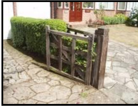
Surviving original gate, post & 'crazy paving' style concrete drive; notice "noughts and crosses" gate design.
