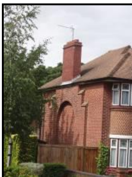
Rustic brickwork with chimney supported by relieving arch, which is all constructed in engineering bricks
