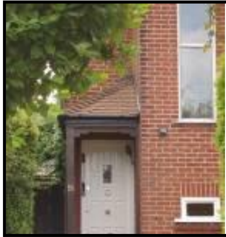
Original side porch with out of keeping replacement door
