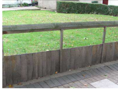
Figure 48: Fence design on Well Hall Road – this is a good copy of the original specification for the Well Hall Road frontages which were designed to a different pattern to the rest of the estate.
