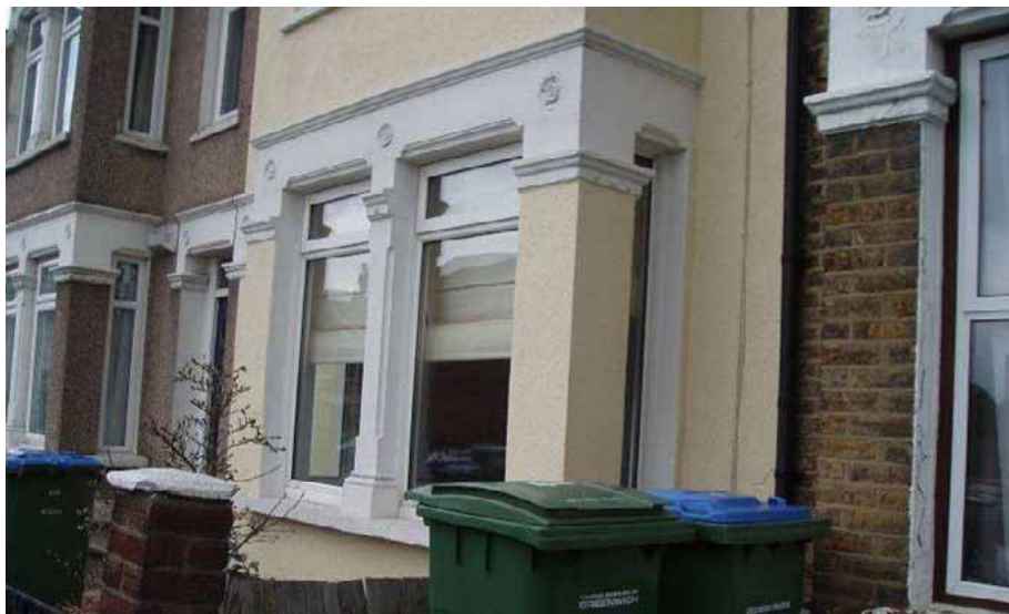
Figure 14: aluminium and UPVC windows, pebble dash and render, disfiguring changes all of which would require permission in the area controlled by the Article 4 Direction.
