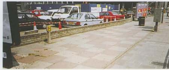
▲ What to avoid Multi-coloured paving pattern poorly designed and built.
