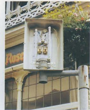
▲ Damaged equipment: the cumulative effect of such damage to equipment can very noticeable, and needs to be kept to a minimum.
