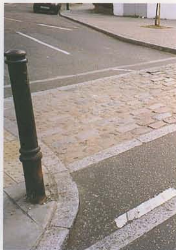
▲ A speed table: using a simple design and good quality materials such as granite setts.
