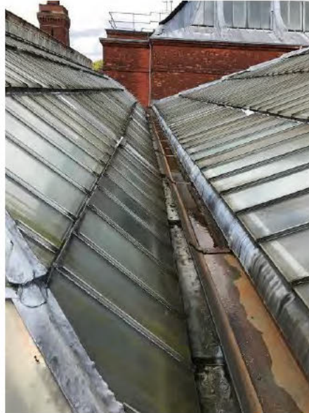
Photo 6 - Roof structure valley gully showing signs of corrosion and in need of cleaning.
