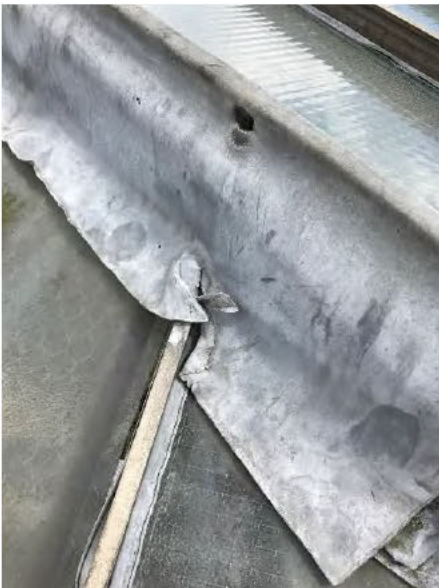
Photo 7 – Fissure to lead capping above glazing bar.
