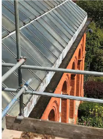
Photo 2 – Lead flashing to roof looks tired and guttering requires cleaning.
