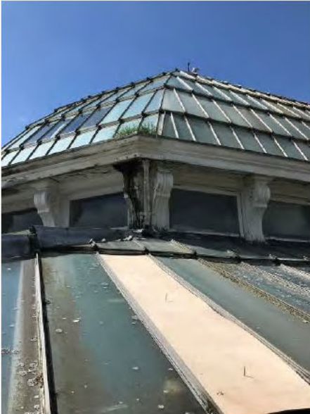
Photo 1 – Rotting timber scrollwork to Temperate cupola roof.
