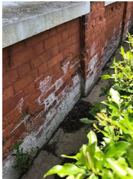
Photo 12 – Minor spalling and efflorescence staining to external brickwork at low level.
