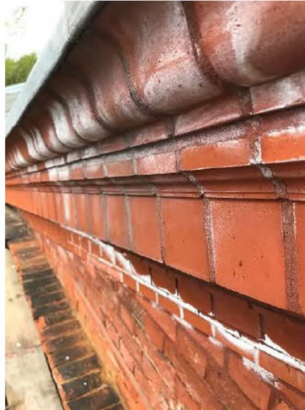
Photo 10 – Efflorescence to high level external brickwork cornice.
