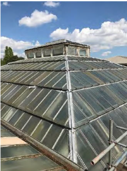
Photo 3 – The Bird Room: Lead flashing on roof structure is loose and hanging off in areas. Rotting timber to cupola roof.
