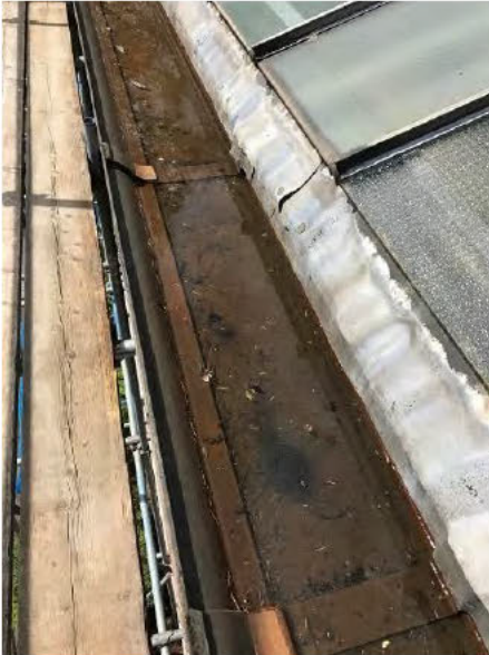
Photo 5 – Roof structure valley gully showing signs of corrosion and in need of cleaning.
