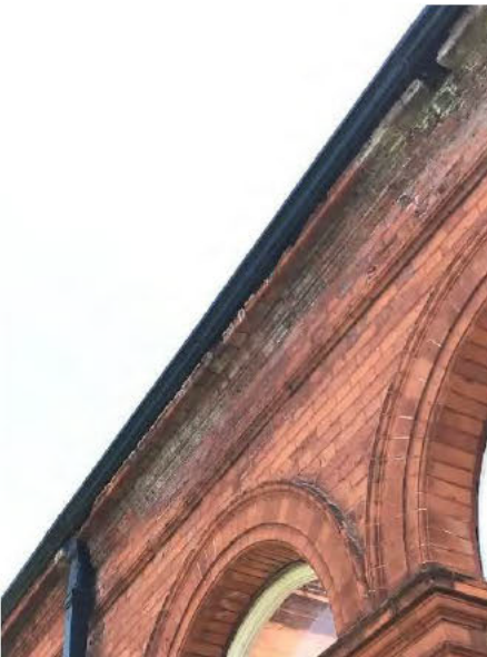
Photo 11 – Algae growth to external walls at high level and underside of cast iron guttering.
