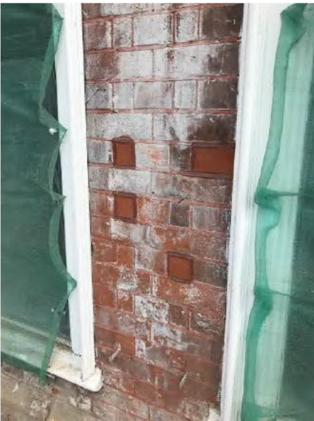
Photo 23 - Efflorescence to Tropical Room wall.
