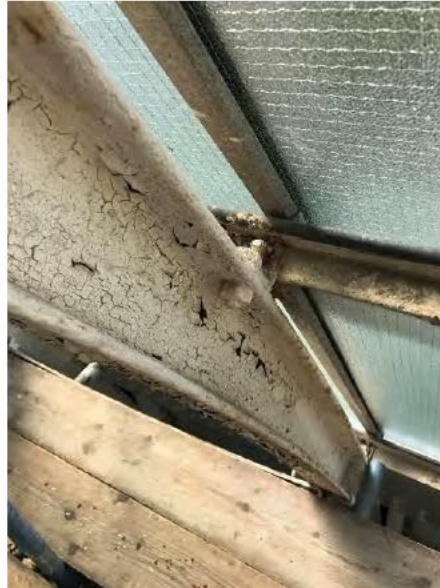
Photo 26 - Flaking paint finishes to iron roofing structure.
