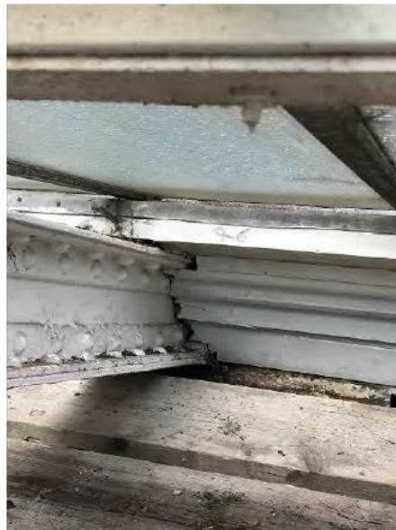
Photo 28 – Rot noted to edge of timber cornice.
