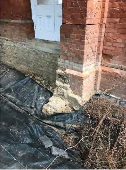
Photo 21 - Damaged brickwork to pillar within the Temperate Room.
