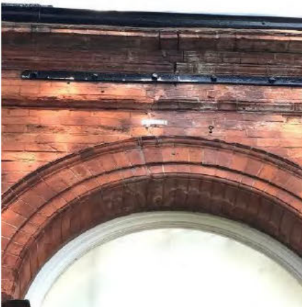
Photo 15 - Stepped cracking to brickwork wall above external window to Tropical Room.
