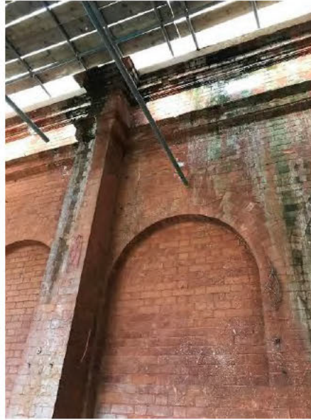
Photo 22 - Algae growth and efflorescence to South wall and pillar within the Temperate Room.
