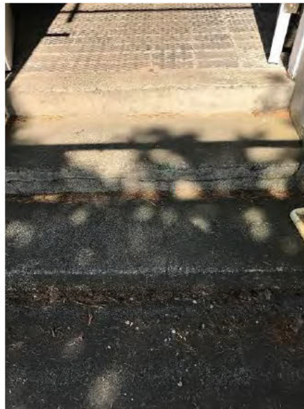
Photo 16 - External steps of main entrance to the Temperate Room cracked and spalled to edges.
