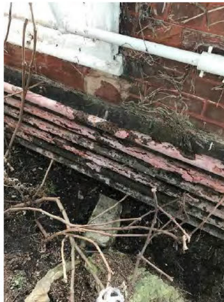
Photo 24 - Flaking finishes to redundant pipework to the perimeter of the Temperate Room.
