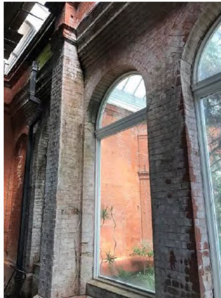
Photo 20 - Extensive efflorescence staining and algae growth to the East wall of the Temperate Room.
