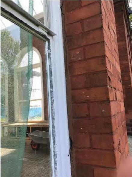
Photo 13 – Cracking surrounding window sub frame. Also flaking finishes to steel window casings.
