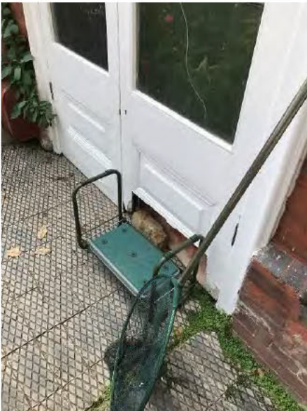
Photo 19 - Door set leading from the Bird Room into the Temperate Room damaged at low level.
