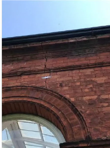
Photo 14 – Stepped cracking to brickwork wall above external window of Tropical Room.
