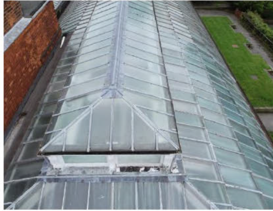
Photo 30 – Timber panel missing to window.
