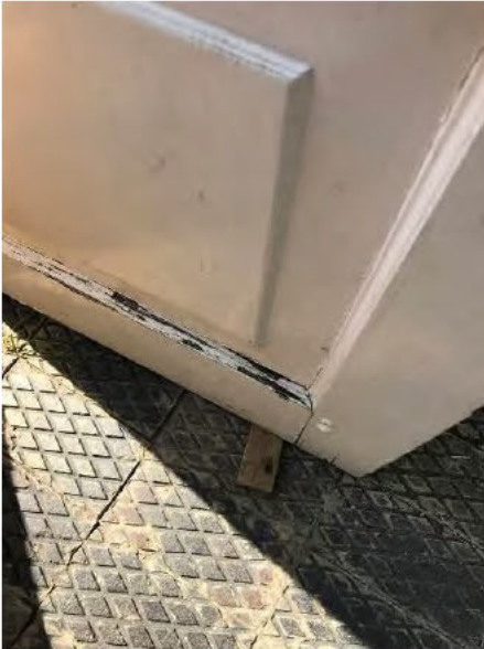
Photo 17 - Rotting timber to Temperate Room main entrance panelled door.
