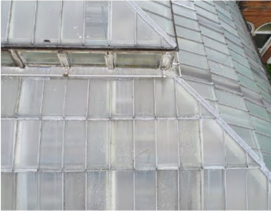
Photo 29 – Timber frame to window rotten.
