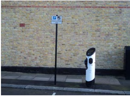
Electric car charging point, Kellerton Road
